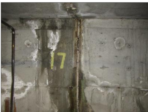
Water ingress on the south portion of the UPG as well as a view of the deteriorated expansion joint in the same location.
