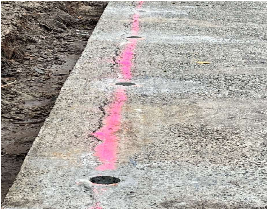
Picture 1: Continuous cracking along basement wall on south
