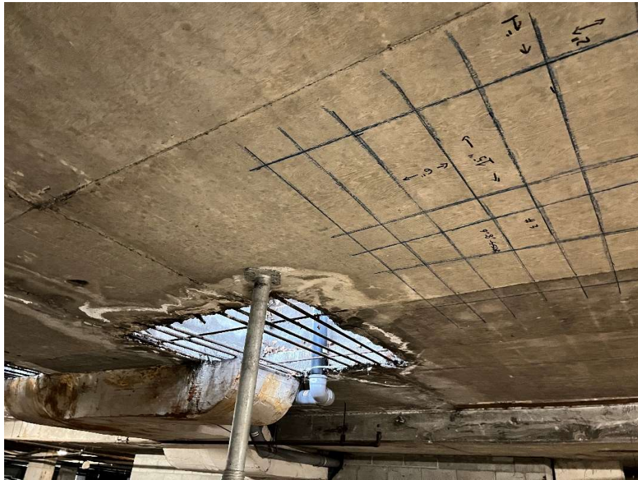
Picture 5: Scanned rebar and exposed rebar
