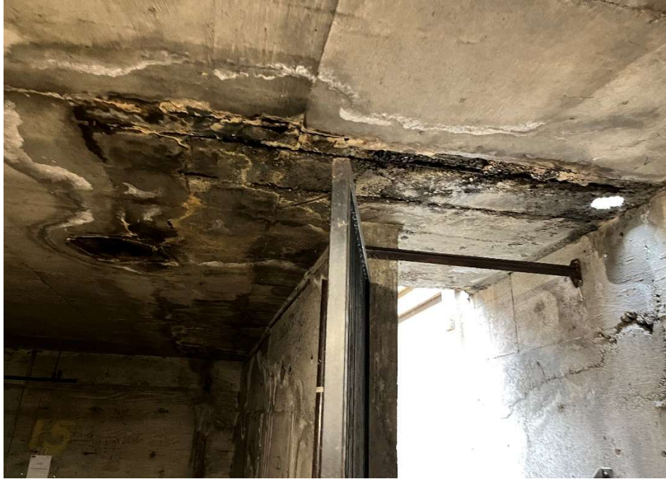
Picture 7: Exposed bottom rebars
