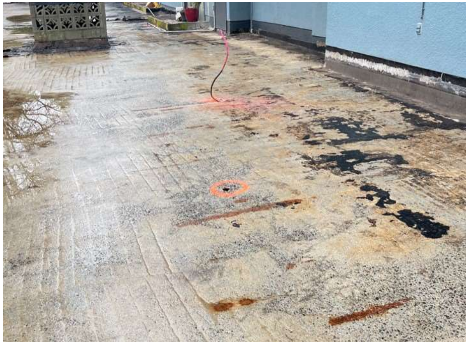
Picture 6: Exposed top rebar
