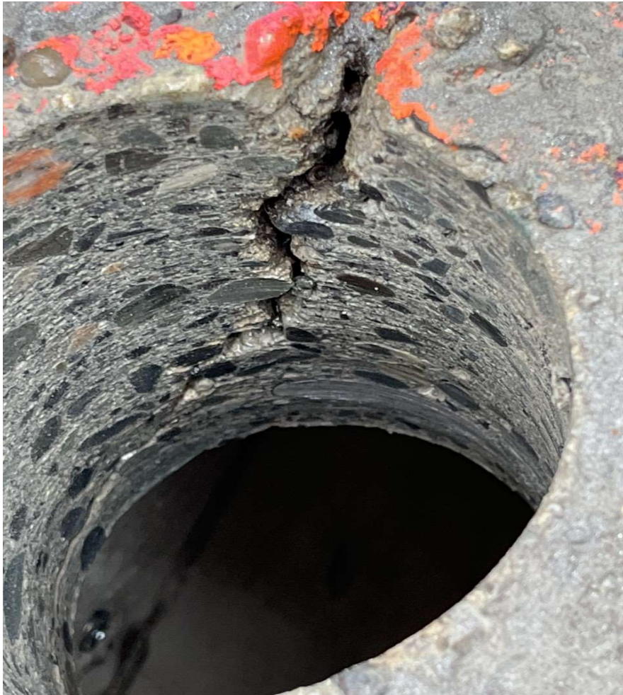
Picture 1A: Cracking observed from core hole
